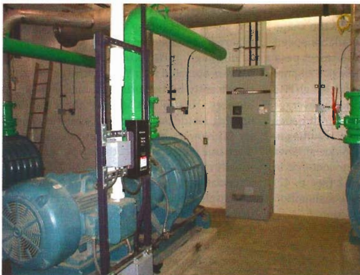
A typical installation of multistage centrifugal blowers with variable-frequency drive control.
